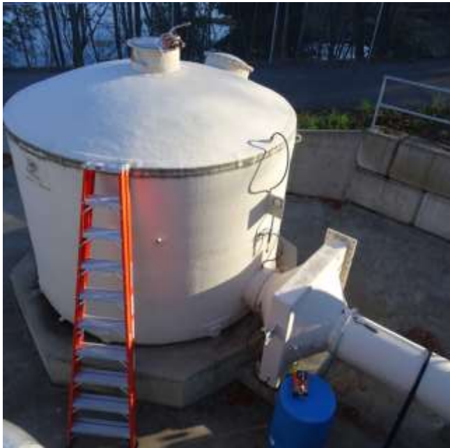
Figure 3. Photo of a carbon filter at a wastewater treatment facility
